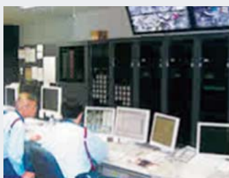
At the disaster prevention center of Daimaru Tokyo store, we centralize control through various monitors to confirm the safety of the whole building.
